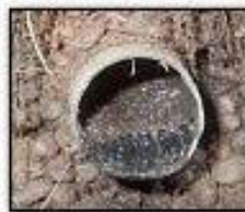
Drainfield pipe plugged with septic tank solids.
