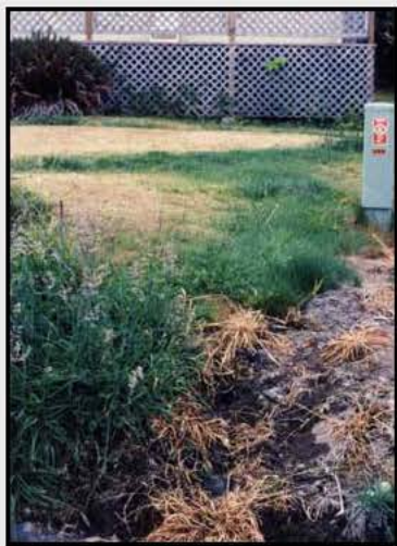
Signs of a failed septic system may include greening grass, saturated soils, and odor.
